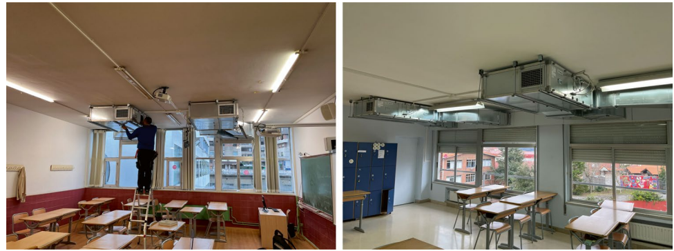
Fig. 6 ESKOaire devices installed at two pilot classrooms. Source The authors
