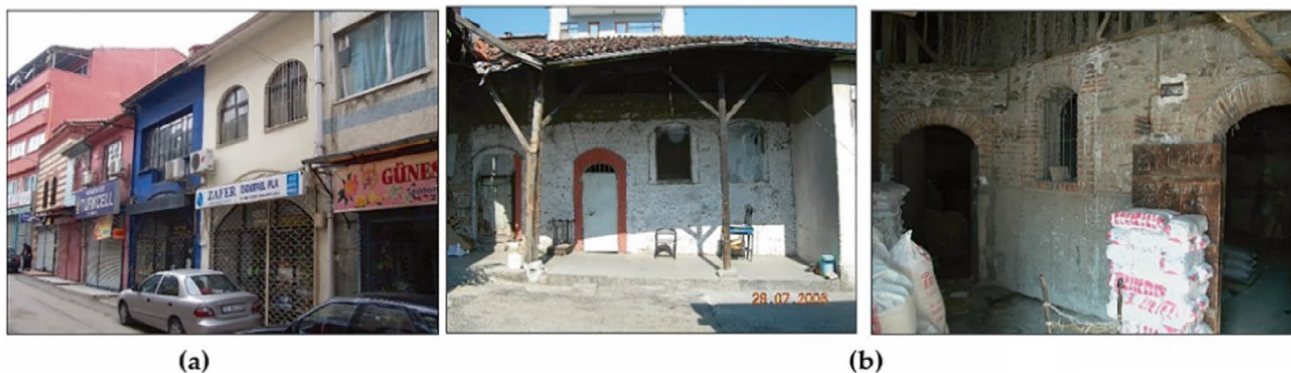
Fig. 3 The traces of historic buildings outside of the boundary of the YGPH: a Five small units of the YGPH built along Çancular Street b photographs of the twentieth-century Ottoman Han newly attached to YGPH from its courtyard (photographed by the Author, 2007)
