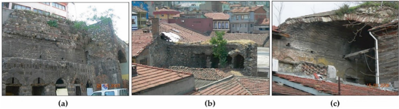
Fig. 2 The existing (and separated) remains of the YGPH a the vaults on the east side of the YGPH; b small rooms on the upper storey and west side of the YGPH; c partially collapsed vault at the southeast corner of the YGPH (photographed by the Author, 2007)
